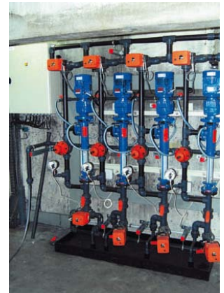
To comply with the tioned specifications, Sodimate selected four reliable, vertically mounted progressive cavity pumps for PAC slurry feeding.
